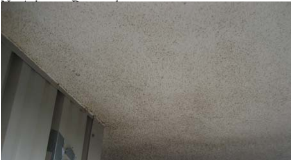
Photograph 3- S001 Textured Ceiling Material Exterior Porch, Level 300
