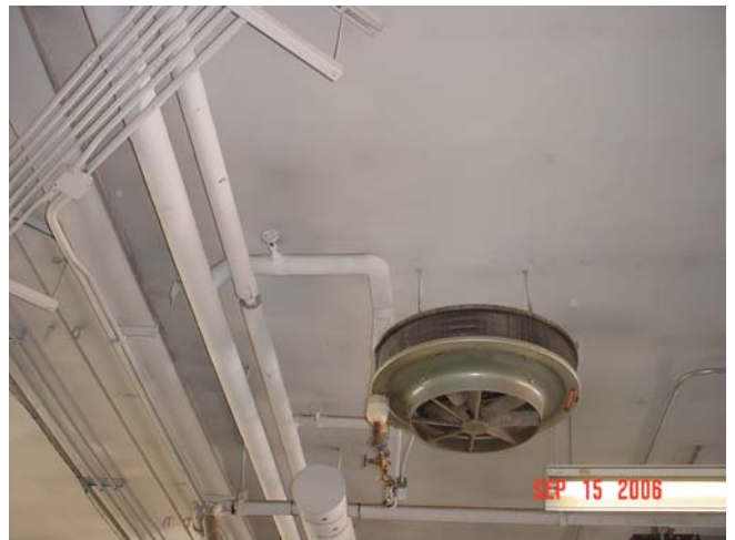
Photograph 4-SUU FACILTITES/AUTO Automotive shop, T001, TSI joints/fittings (mudded, ACM).
