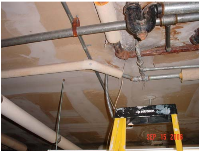
Photograph 3-SUU FACILTITES/AUTO Room 001, T001, TSI joints/fittings (mudded, ACM).
