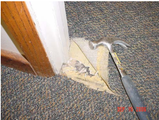
Photograph 5-SUU FACILTITES/AUTO Facilities building, main hallway, M002 9" floor tile under carpet, ACM.
