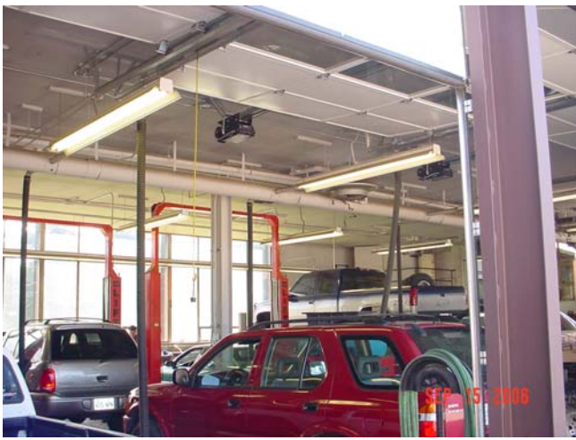
Photograph 7-SUU FACILTITES/AUTO Auto shop, T001, TSI joints/fittings-mudded, ACM.
