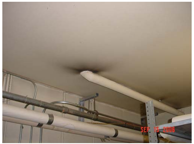
Photograph 2-SUU FACILTITES/AUTO Room 002, T001, TSI joints/fittings (mudded, ACM).
