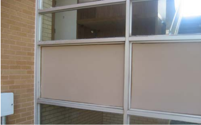
Photograph 1- M007 Window Caulking Exterior Windows Contains 5% Asbestos & LBP
