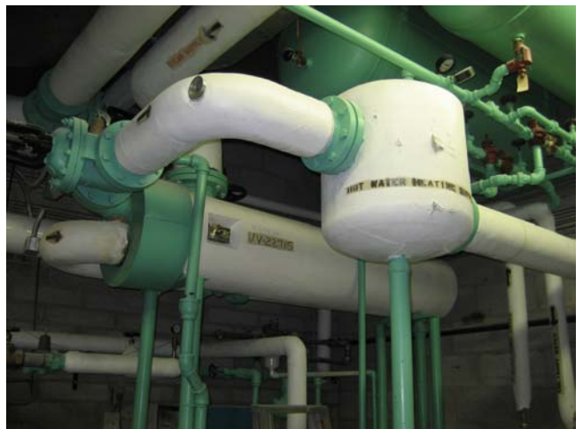
Photograph 6-SUU MUSIC BUILDING Room 110, Mechanical room, T002, Asbestos heat exchanger (background, horizontal). Up from the floor ~7 feet.
