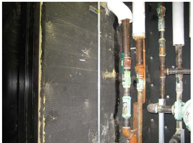
Photograph 4-SUU MUSIC BUILDING Room 110, Mechanical room. Asbestos Acoustical Liner (T001).
