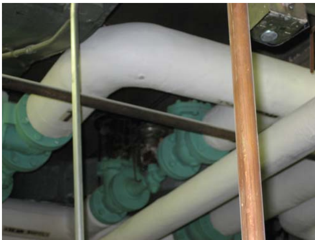
Photograph 9-SUU MUSIC BUILDING Room 111, Mechanical room with Asbestos TSI joint/fittings-mudded.
