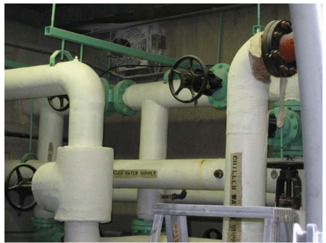
Photograph 8-SUU MUSIC BUILDING Room 111, Mechanical room with Asbestos TSI joint/fittings-mudded.
