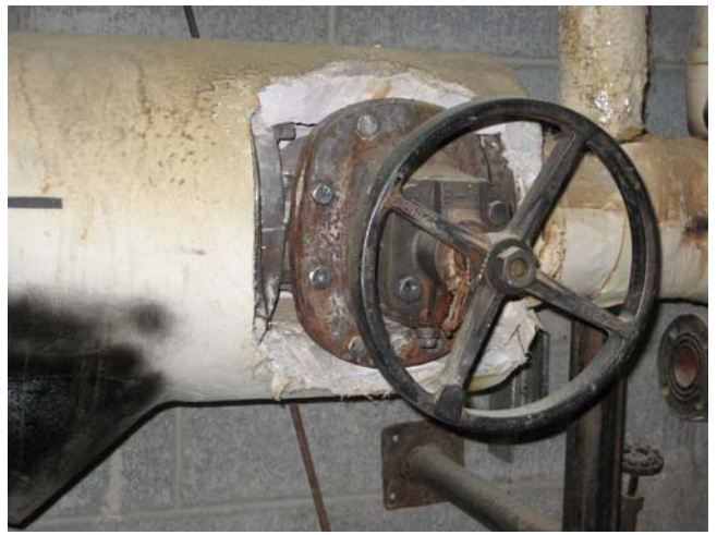
Photograph 14-SUU MUSIC BUILDING Room 111, Asbestos TSI valve body.
