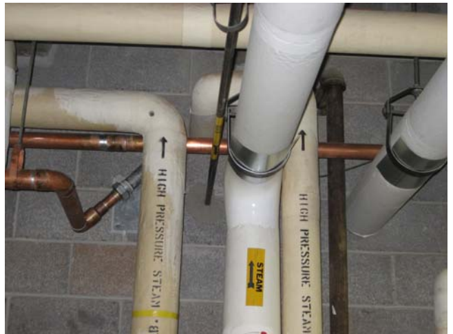
Photograph 16-SUU MUSIC BUILDING Room 111, Mechanical room with Asbestos TSI joint/fittings-mudded.
