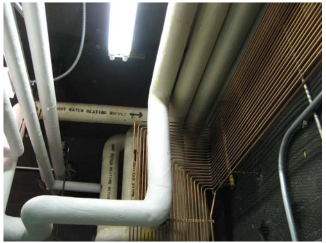
Photograph 2-SUU MUSIC BUILDING Room 110, Mechanical room. Asbestos TSI joint/fittings-mudded. Pipe lagging straight runs are fiberglass insulation.
