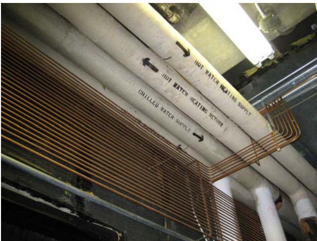
Photograph 3-SUU MUSIC BUILDING Room 110, Mechanical room. Asbestos TSI joint/fittings-mudded (T002). Pipe lagging straight runs are fiberglass insulation.
