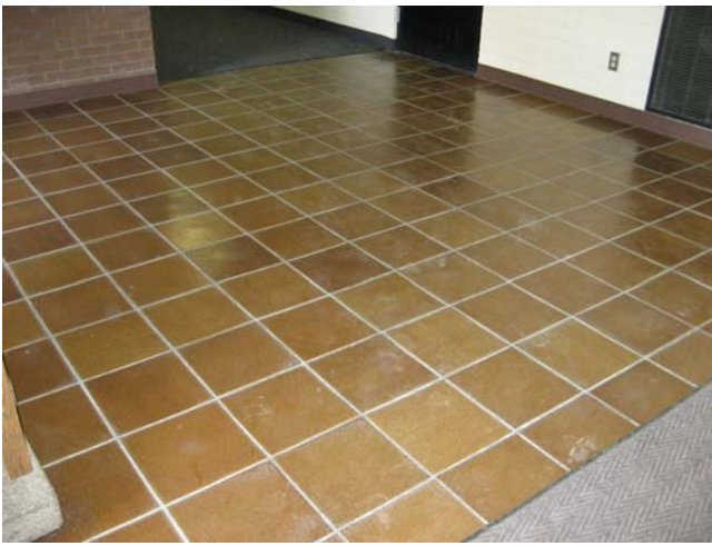
Photograph 13-SUU MUSIC BUILDING Front entry ceramic tile, Lead containing glaze.
