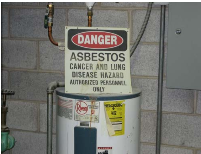
Photograph 7-SUU MUSIC BUILDING Asbestos sign in Room 110, Mechanical room.
