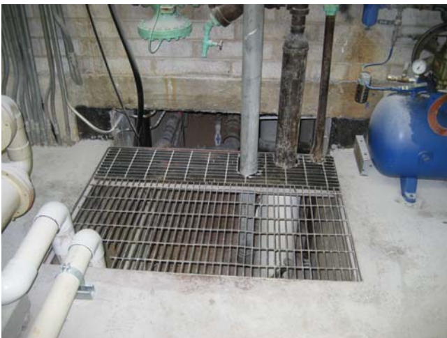
Photograph 5-SUU MUSIC BUILDING Room 110, Mechanical room, tunnel from Central Heat Plant.
